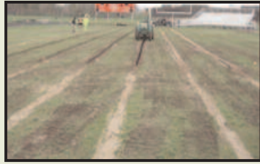
May 2007. Cutting drain lines, installing drain tiles, and backfilling lines with a sand-based root zone material, Grand Blanc High School, Grand Blanc, Mich., Water Management Inc.,
